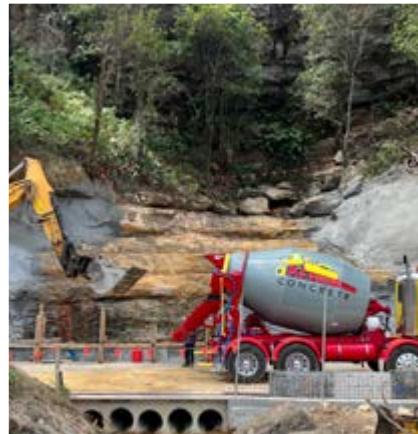
Construction of the temporary bridge on Settlers Road, bypassing the under repair Thomas James Bridge
