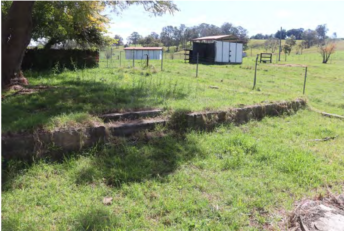
Plate 3-14: Stone retaining wall and steps. Note masonry from fountain in lower right of frame (AECOM, 2022)
