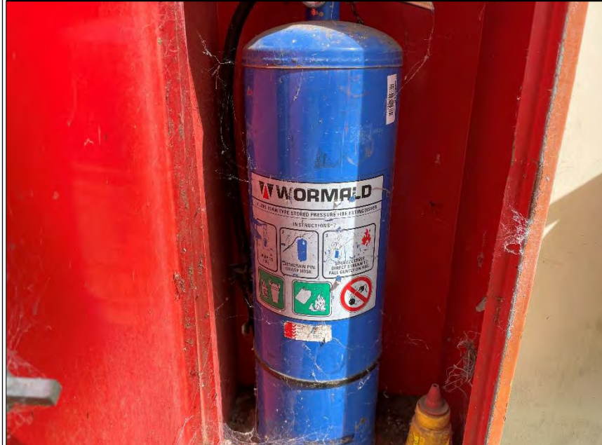
PHOTO 16: AFFF (PFAS) FIRE EXTINGUISHER.
