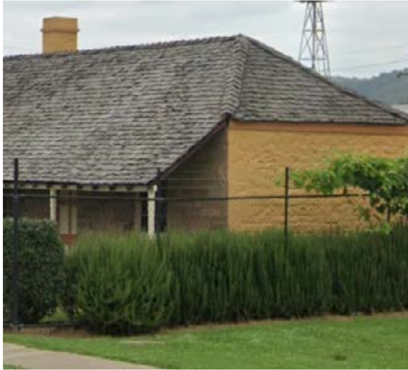
Example of a timber shingle roof, Arms of Australia Inn, Emu Plains
