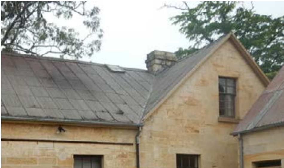
Example of 'Morewood and Rogers' roofing tiles at Woodford Academy at Woodford NSW
