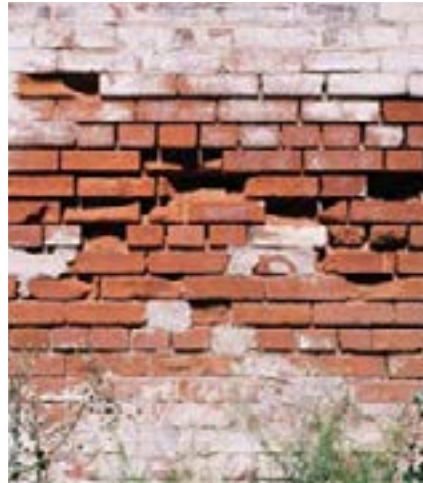
Figure 2: Typical salt damp damage causing decay of the bricks (Heritage Council NSW)
