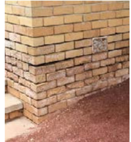
Figure 3: Loss of mortar in joints due to salt attack causing dislodgement of bricks, with white deposits
