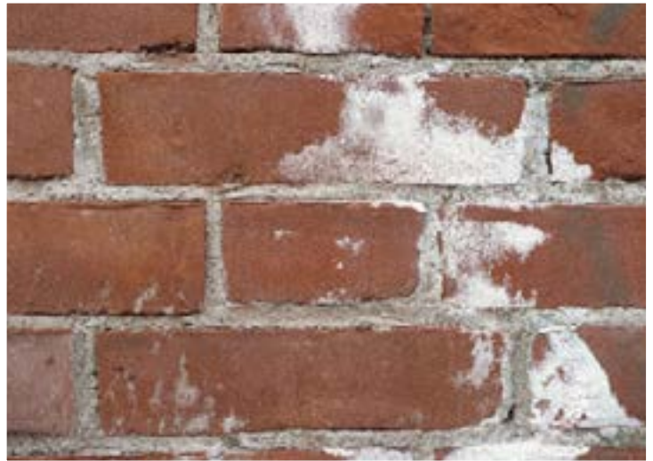
Figure 6: Efflorescence on brickwork caused by the presence of crystalline salt
