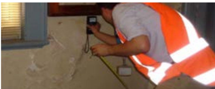
Figure 10: Measuring damp levels in wall with moisture meter
