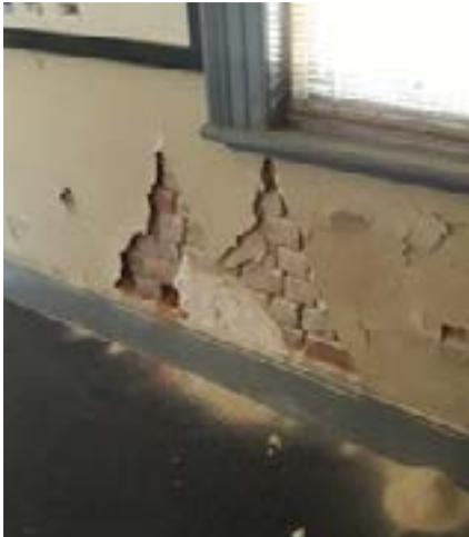
Figure 1: Typical blistering of paint and damage to plaster finish caused by combination of rising damp and salt
