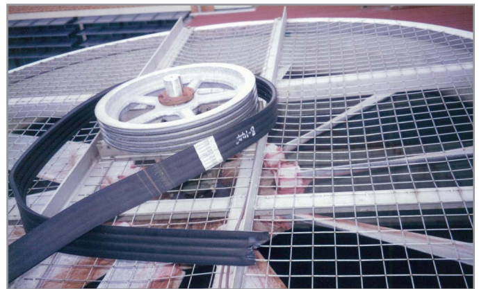
Figure 5.4-1: Broken fanbelt where the motor functions but the fan does not
