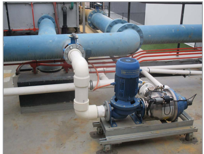
Figure 5.1-3: Side stream filtration equipment at the balance line, connecting three cooling tower basins
