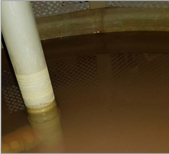
Figure 5.3-1: Cloudy or discoloured cooling water can indicate poor water cleanliness or insufficient cleaning and servicing
