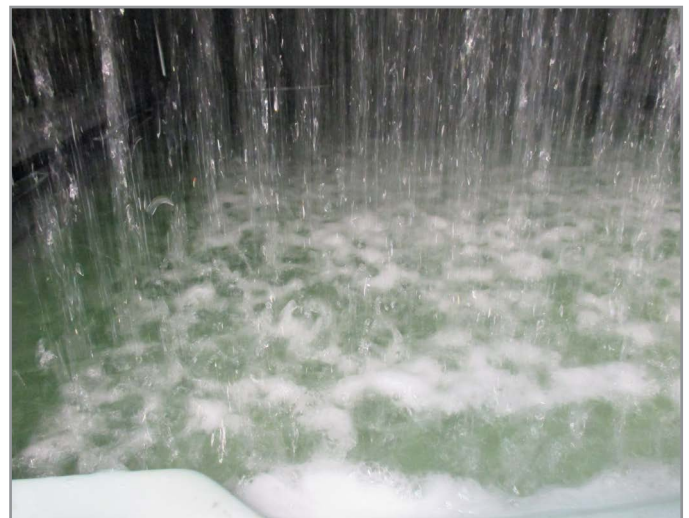
Figure 5.1-4: Even fall of water across basin area suggests fill passages are clear
