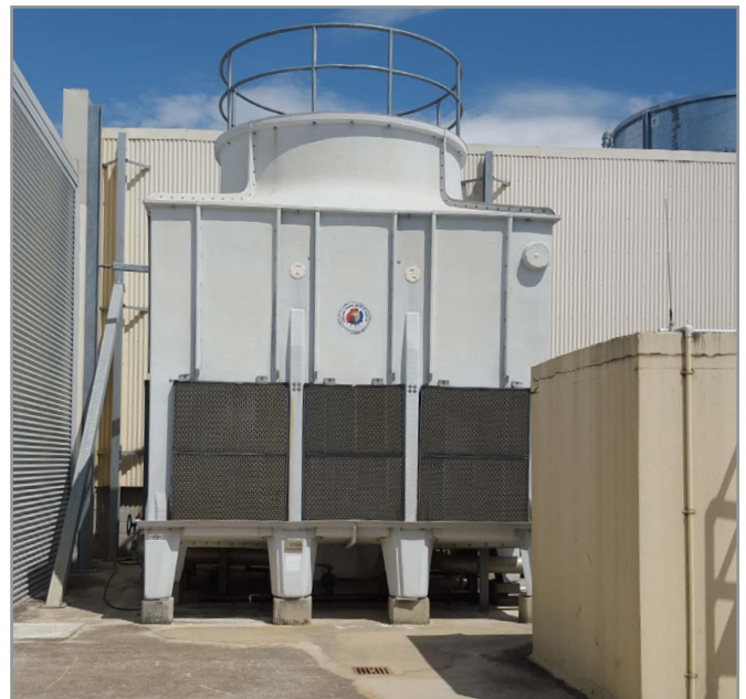
Figure 5.5-2: A cooling tower with no walkway or platform to allow removal of access panels for inspection and maintenance
