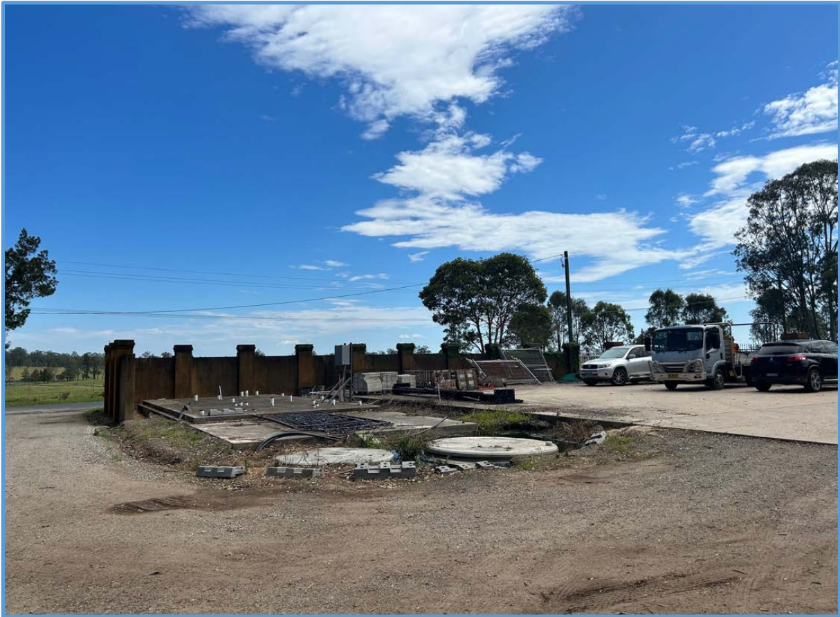
Figure 10: Existing, unauthorised slab illustrating pipe penetrations.
