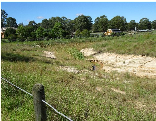
View east from Bootles Lane of eroded northern drainage line
