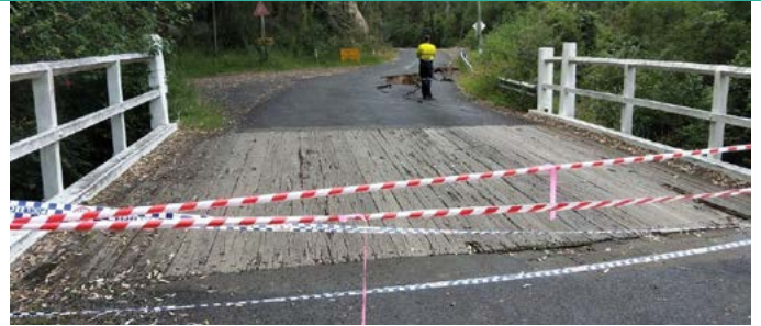
Thomas James Bridge, Settlers Road damage
