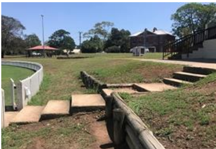
Photo 12: Slope between grandstand and oval showing erosion and poor seating options – refer to proposed works (3/02/2020).
